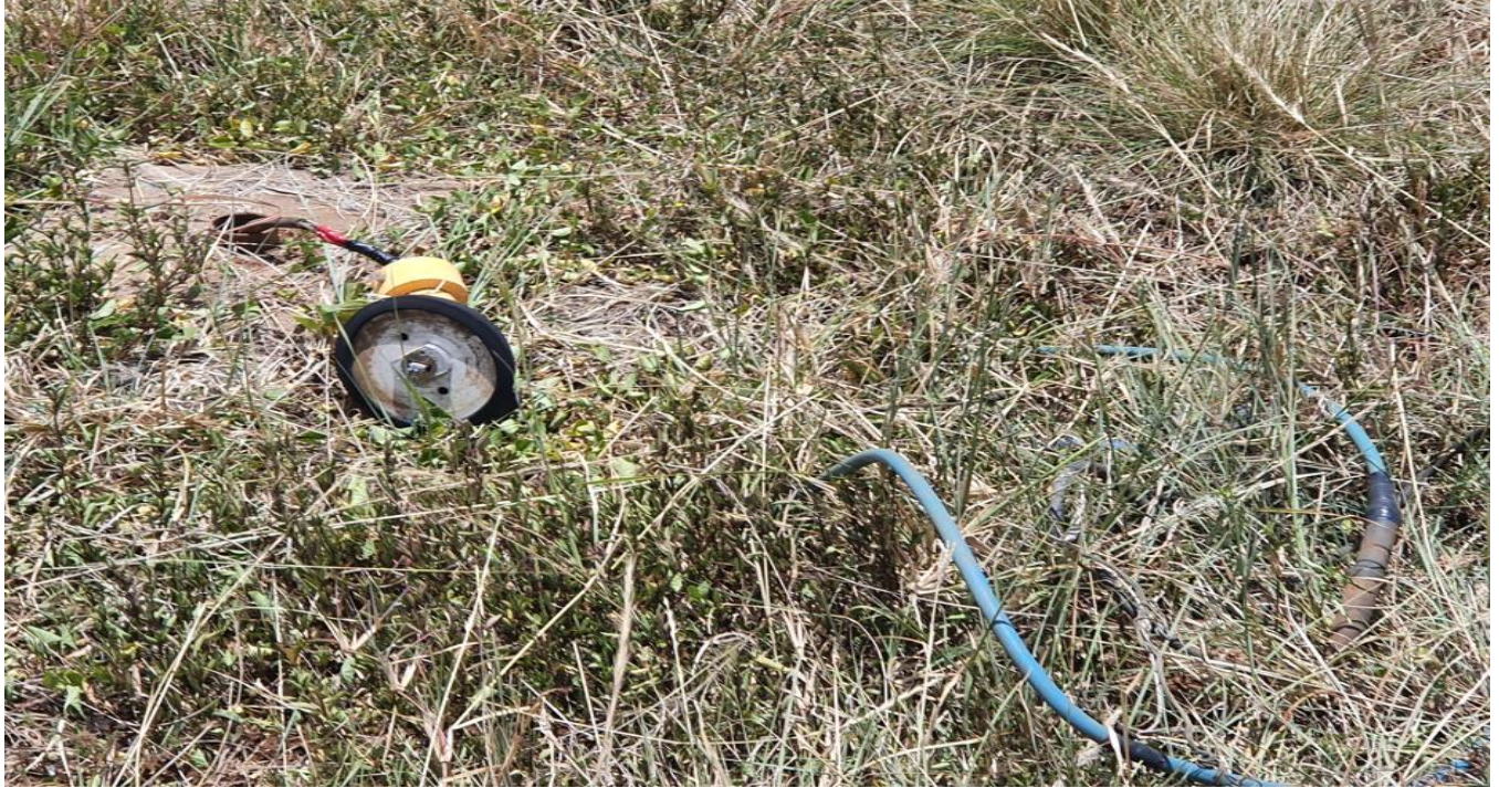
Fig 2: Damage on the runway edge light
